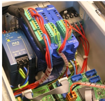
... and fits in every control cabinet (pictured with two extension moduls) including a total of up to 14 outputs.
